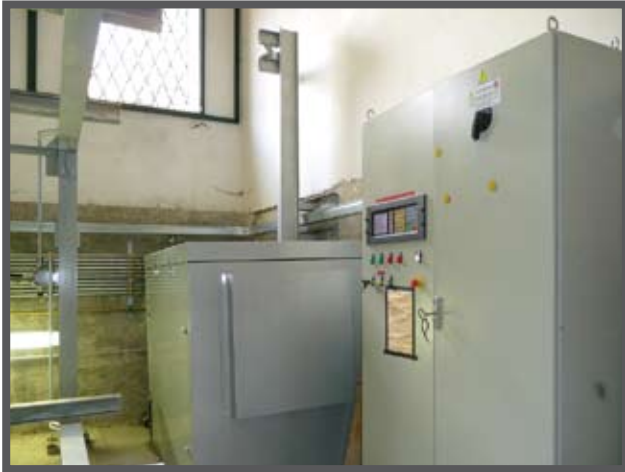
Fig 4: View of the hydraulic lift control unit complete with protection casing and control panel with interface for monitoring, alarms and maintenance of the systems.
