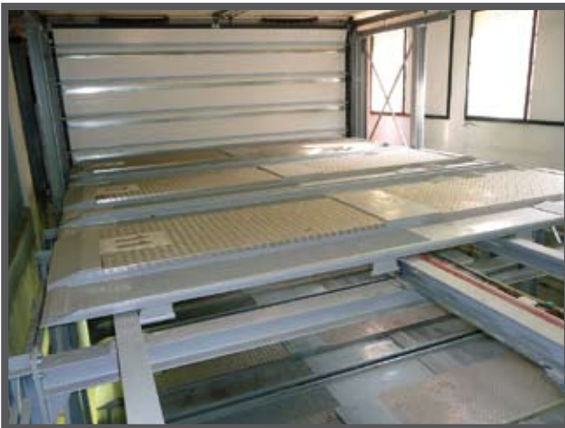
Fig 3: Area beside the entrance where the vehicle platforms are stored showing the sectional door closed.
